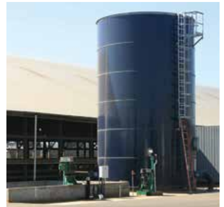
Right: Flush management of parlor, holding pen and special needs barn on a 3,000 cow scrape dairy in Western Washington.
